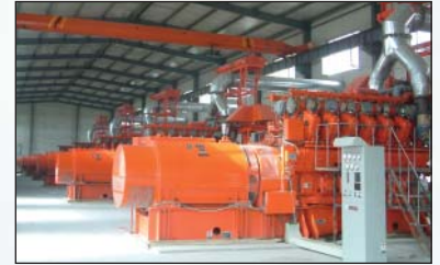
At a privately owned power plant in Kashi, China, six Waukesha 12VATGL gensets supply heat and electricity to residential and business customers.
