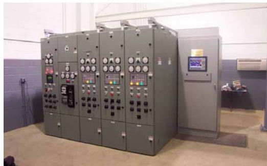
Control Room Switchgear
