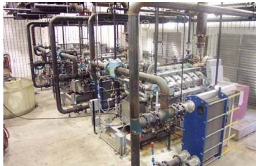
Waukesha 7100 GSI Engine Units
