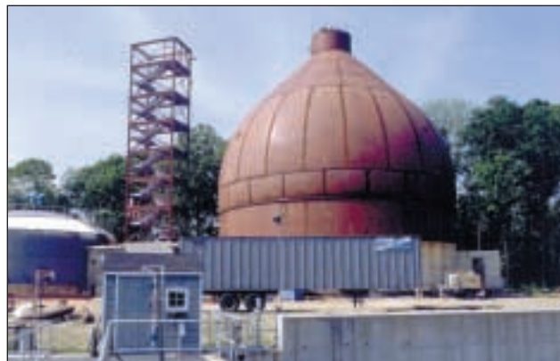
The anaerobic "egg" sludge digester
